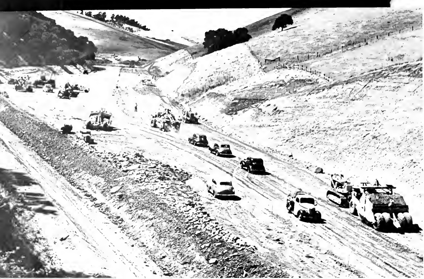
Equipment working on new grade of relocated Franklin Canyon highway. Channel change of Franklin Creek below level of old road shown at left
